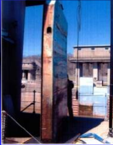
Current steel panels
