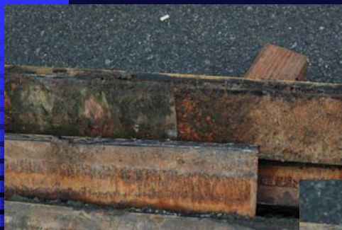
Very corroded existing steel blocks.
